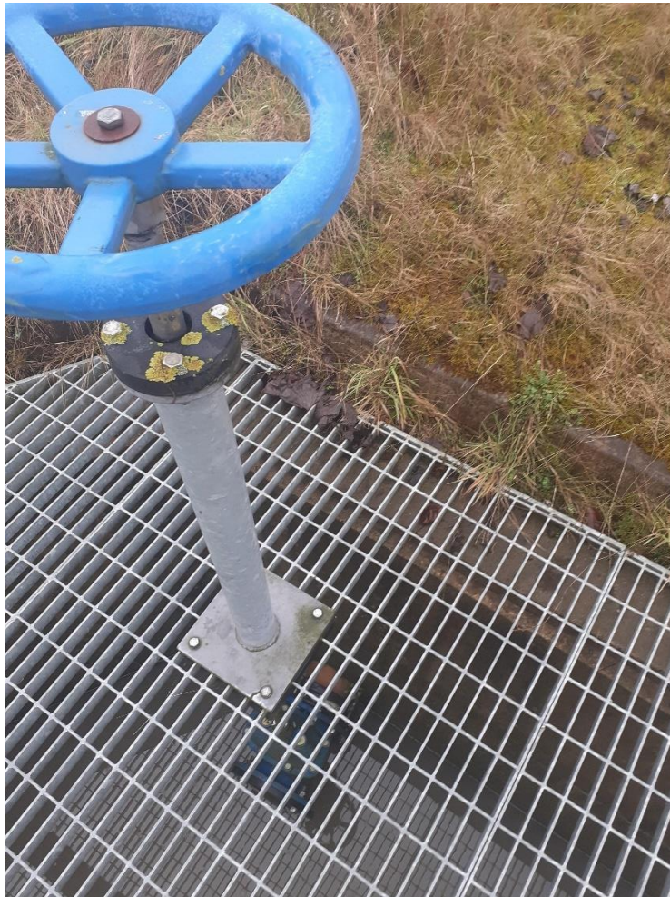
Figure 5-3 Gate Valve in Concrete Tank
